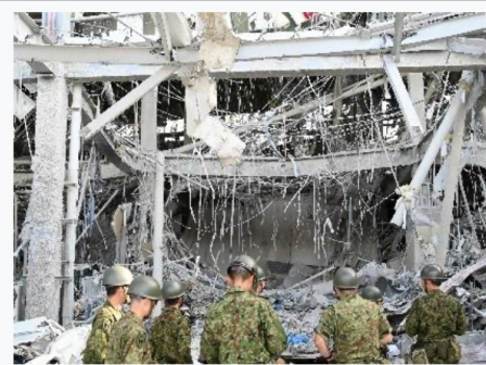
JGSDF personnel inspecting the partially collapsed AEON Mall Kumamoto in Kashima
